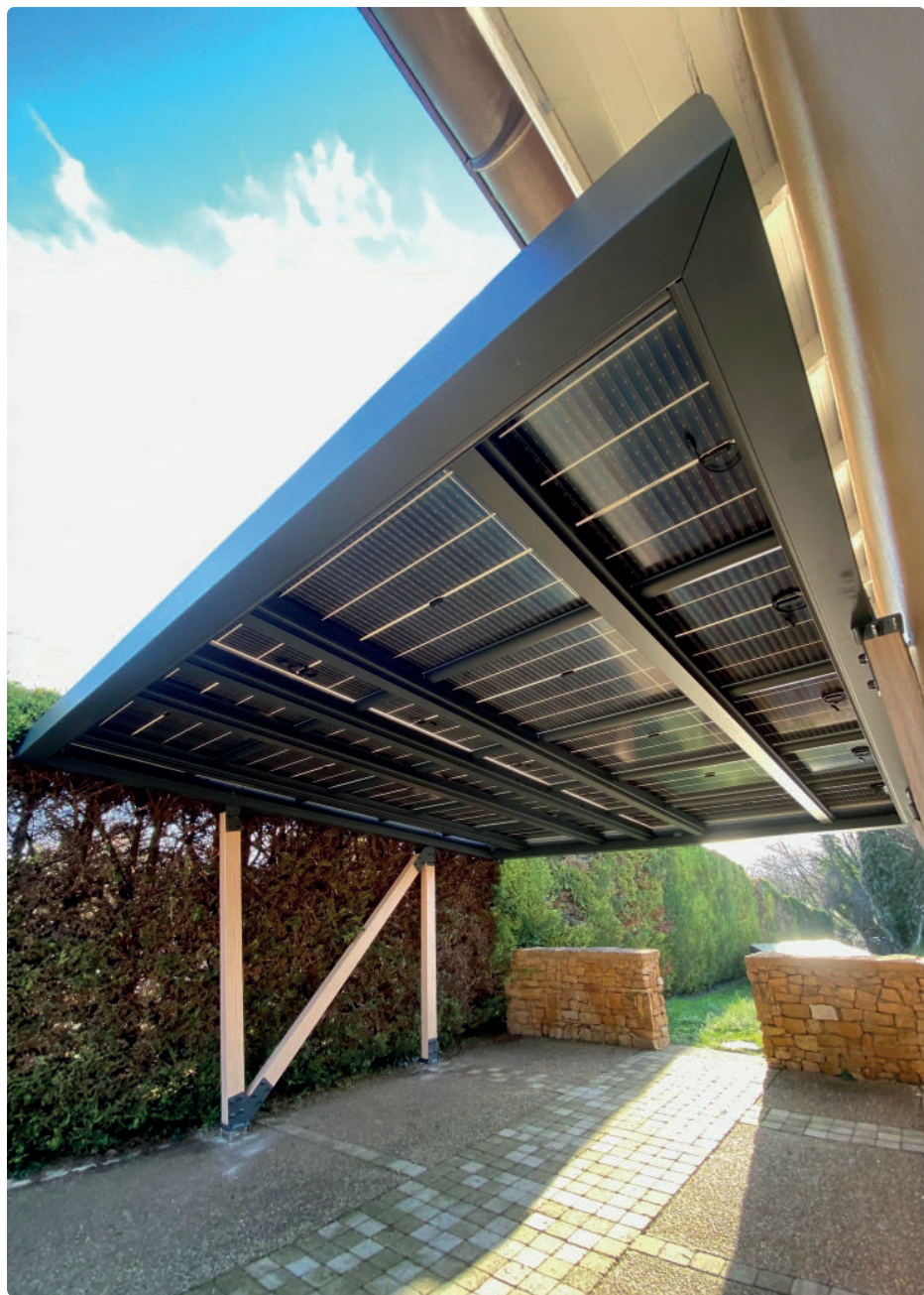
Installation 6 kWc - 2 places
